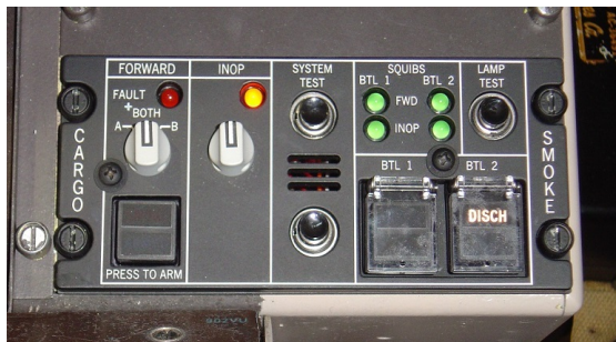
Fire Suppression Control Head
